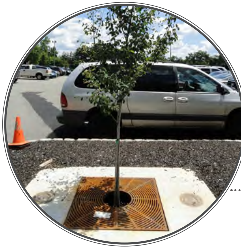
LOCATION: Parsippany, NJ This enhanced tree pit is located at the Parsippany-Troy Hills Municipal Court parking lot. The tree pit collects and filters water from the existing parking lot.
