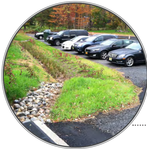
LOCATION: Parsippany, NJ This bioswale was installed at St. Gregory's Church. The bioswale was designed to capture water from the parking lot and move it toward the forest area on the south end of the site.
